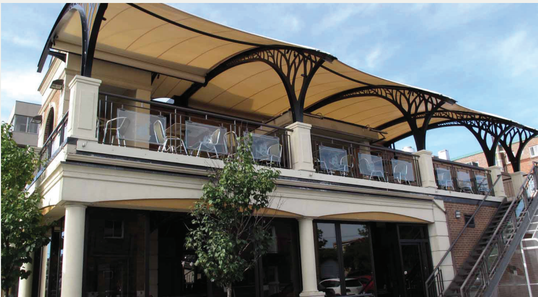
Arch anchoring to existing building differs from one arch to the other
